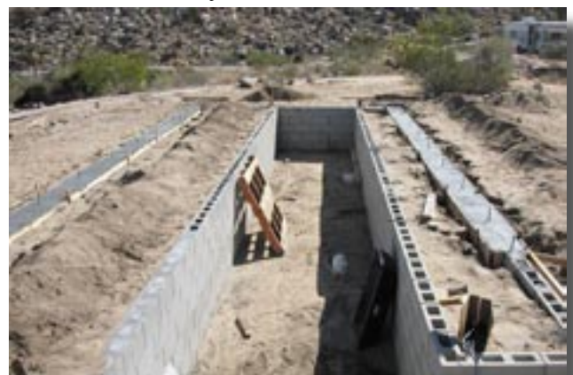
View of the Carbarn Pit with newly poured foundation walls on each side.
