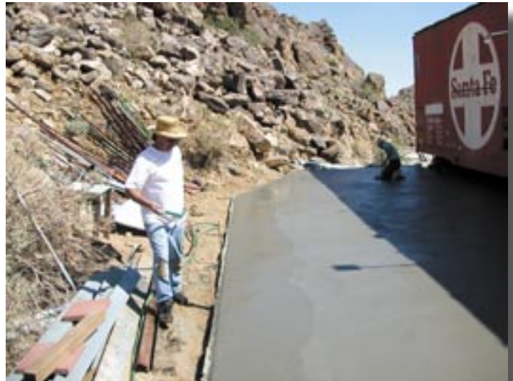
Paul Lavacot wets down the fresh concrete at the Shop Car slab, while Bill Shepard starts on the second pass of finishing.
