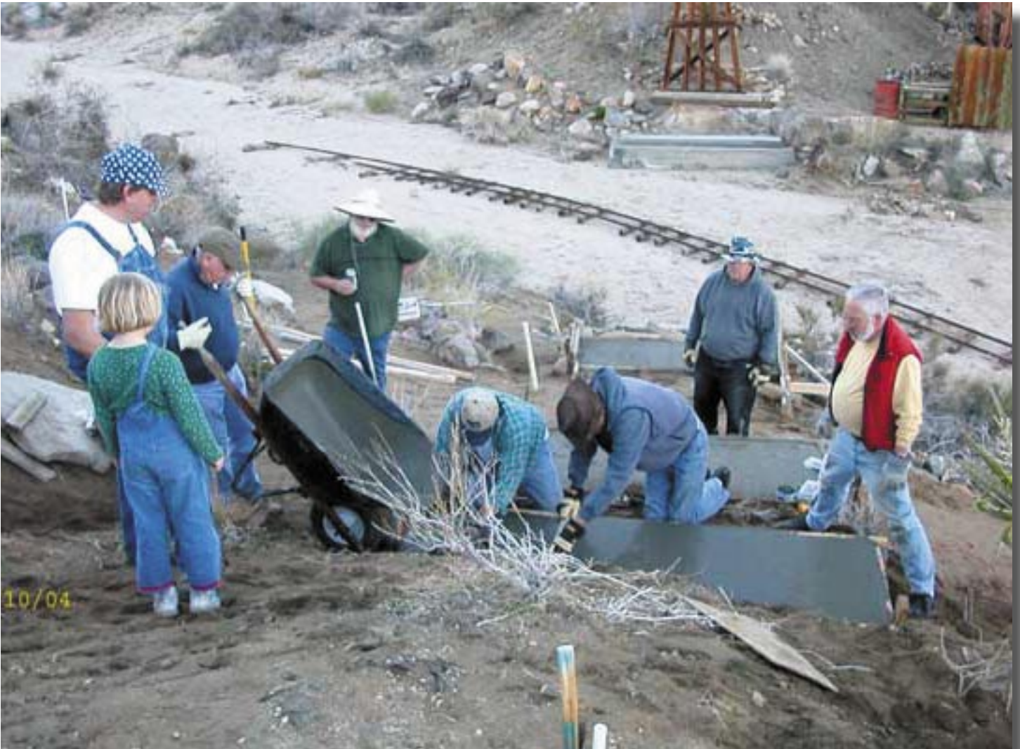
Tom Arnold is dumping the last load of concrete for the day, at the GSD January workday. Paul Lavacot and Jack Sessum are finishing, while Chris and Emily Allan, Lars, Ken and Don admire their work. This leaves only one more footing to pour for Bridge 1.
