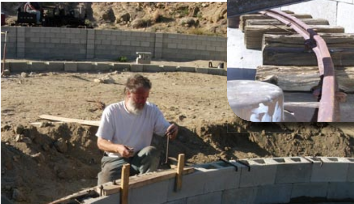
Bill Shepherd placing bolts in the 15" gauge turntable pit wall he constructed.
