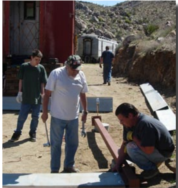
Joseph, Dick and Mike bolt together the framework for the new shelter at the Pullman.
