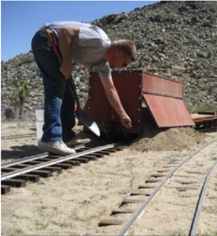
Greg Ratliff takes care of some ballasting chores during the Easter work weekend..
