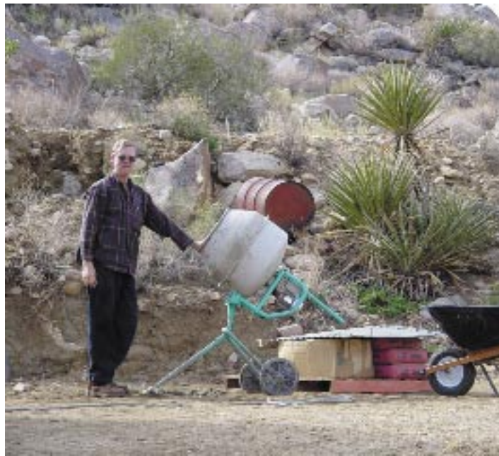
Rick Mugele mans his "batch plant" for the 15" gauge bridge footing concrete pour.
